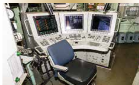
Figure 3. The Integrated Machinery Control System console designed for the Halifax -class frigates.
