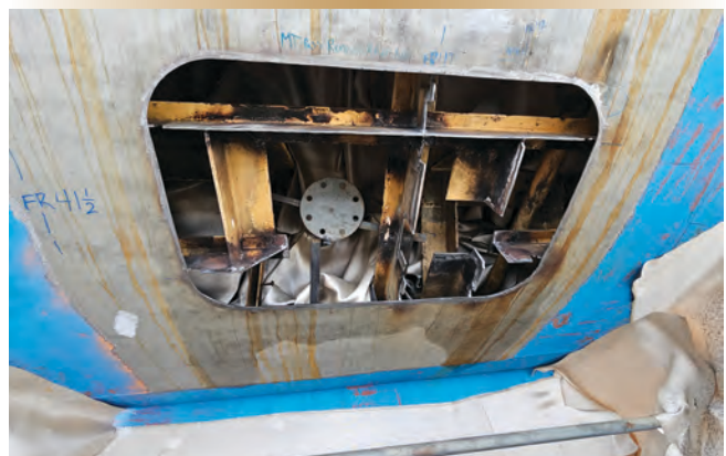
Figure 1. PEC scanning technology offers insight on the state of corrosion in hard-to-access areas of ship structure, allowing maintenance personnel to know which sections need to be opened up for repair.
